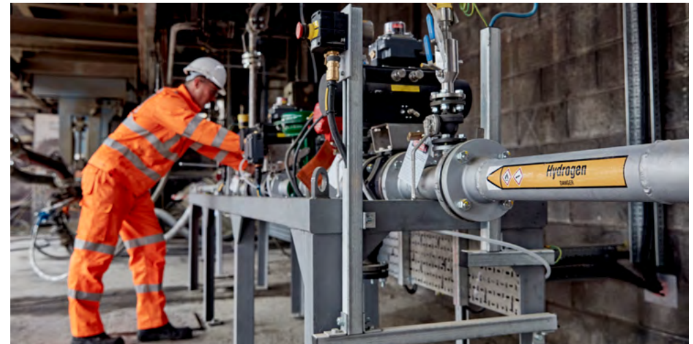
A cement kiln at our Ribblesdale works was successfully operated using a net zero fuel mix as part of a world first demonstration using hydrogen technology.
