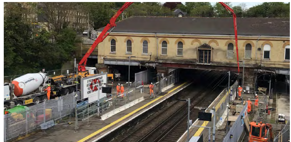
UK's largest single pour of an innovative new cement-free concrete at Chatham Station in Kent.
